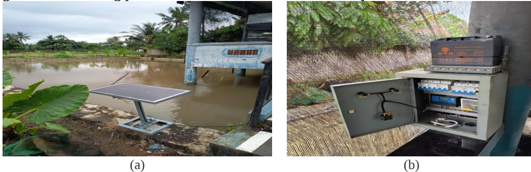
Gambar 7. (a) Solar Panel, (b) Panel Power
